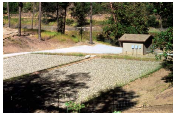
20,000 gpd recirculating sand/gravel filter (RSF/RGF). Packed media filters were found to be a reliable and cost-effective method for achieving secondary or advanced treatment. Systems using attached growth/fixed film processes also tended to have significantly lower power and operational costs as compared with activated sludge processes. Courtesy of Orenco Systems, Inc.
