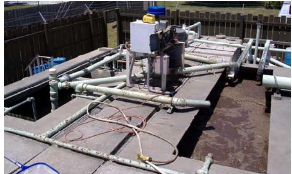
10,000 gpd activated sludge (extended aeration) treatment plant serving a mobile home park. Most large scale decentralized systems studied in Florida and Texas used some type of activated sludge process. Courtesy of state regulatory staff, Florida.
