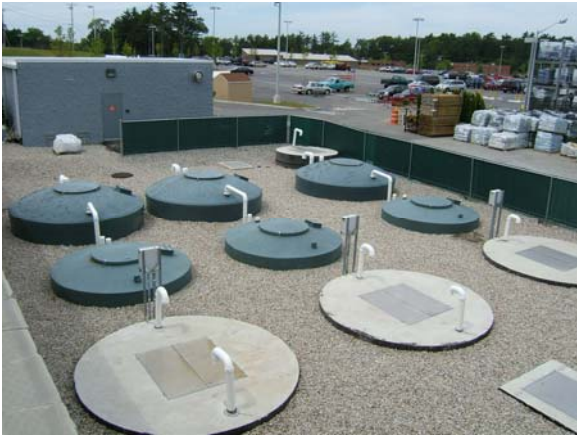
40,000 gallon per day Bioclere treatment system serving a shopping center. This is a proprietary recirculating trickling filter system, and is an example of an attached growth/fixed film treatment process. Courtesy of Aquapoint, Inc.
