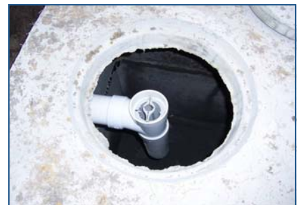
Effluent screens must be accessible for maintenance.
