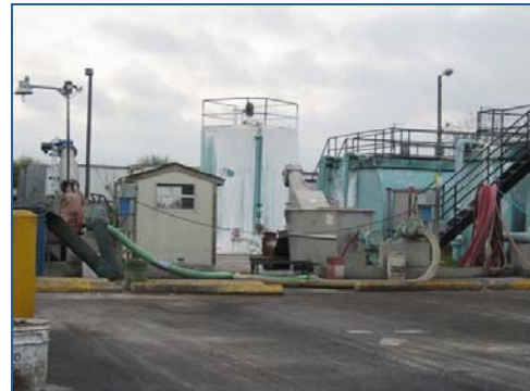
Municipal wastewater treatment plants can accept residuals if there is adequate capacity.
