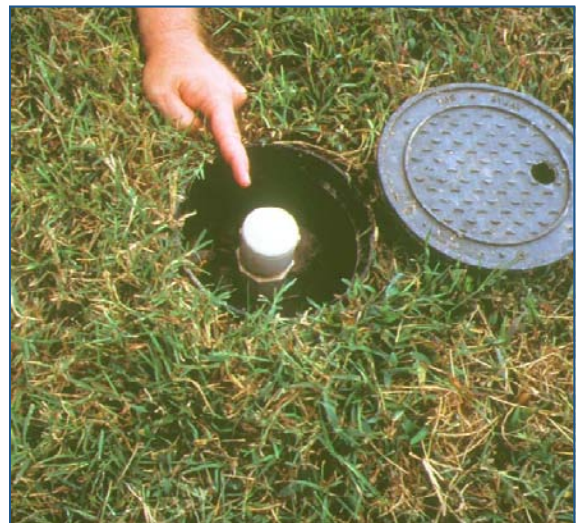
Clean-out with a cap installed in a valve box at the end of an LPD lateral
