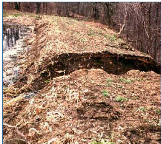
Dike failure may result if appropriate vegetation is not maintained.
