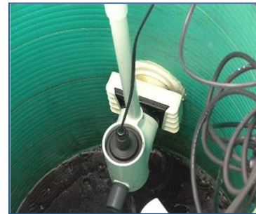
UV light unit installed inside the riser of a dosing tank
