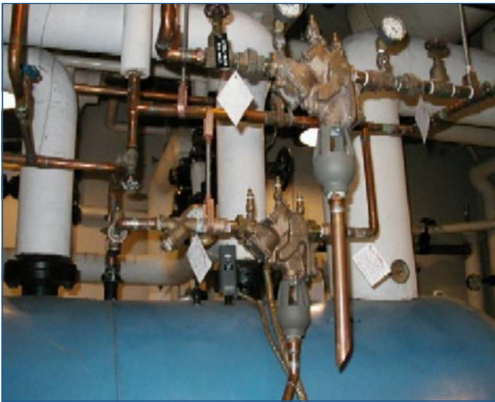
Backflow preventers (in foreground) are required to prevent cross-connections between potable and non-potable water.
