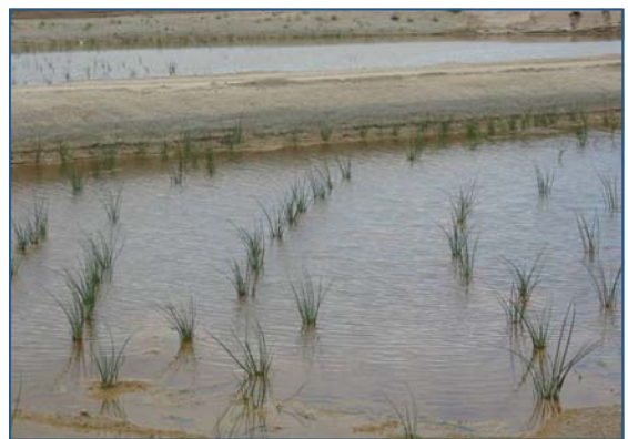
Once it is constructed, locally hardy, non-invasive plants such as bulrushes are established in the cells.
