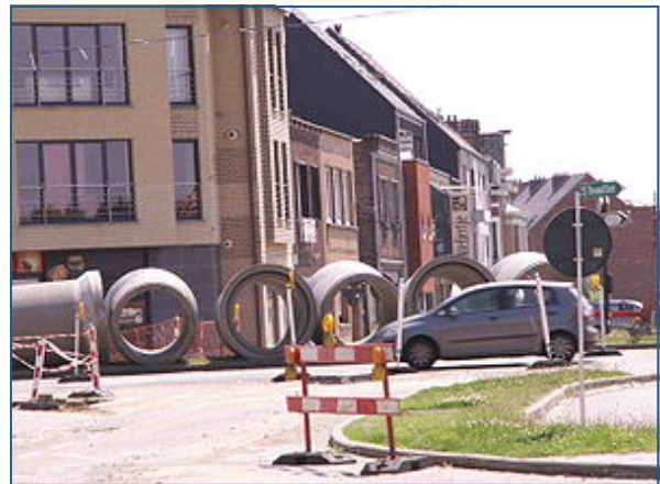
Larger flows require larger diameter pipe for gravity sewer systems. Deeper (and more expensive) excavation is also needed but the cost may be offset by the fact that pumps and lift stations are only required in areas with inadequate slope for gravity flow.
