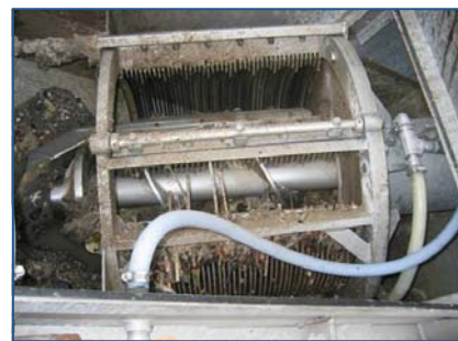
Residuals can be added to a WWTP upstream of screening and grit removal components.
